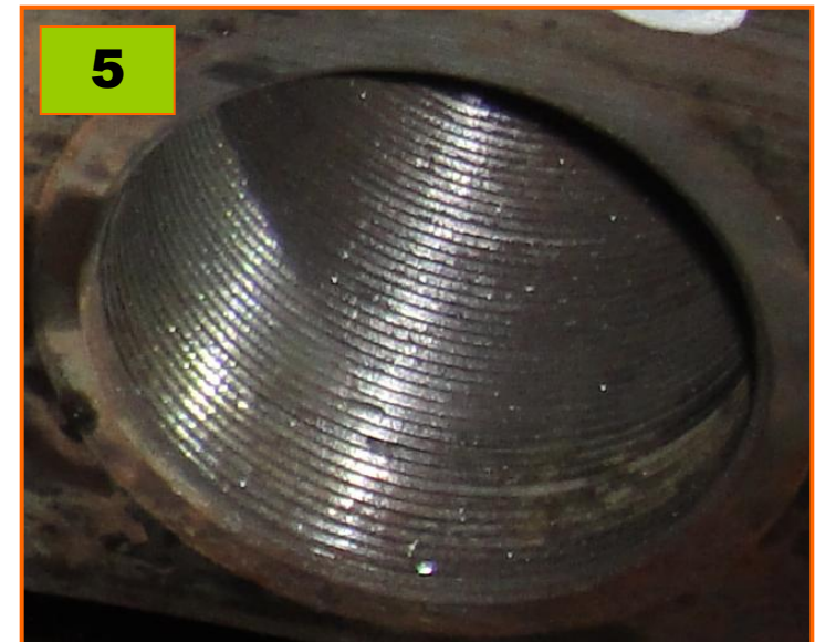
Pic.5 Threading belonging to the pump body after the removal of the stud ends
